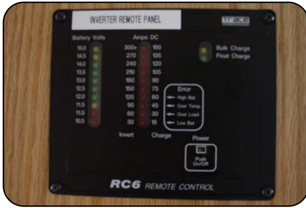
R6 Inverter Charging Panel
